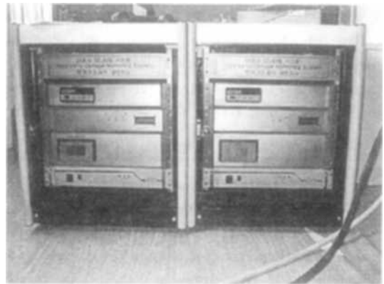
Fig. 6 Developed third-party damage monitoring system
